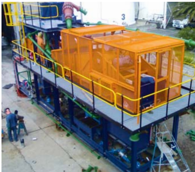
DMS plant at Mandala
